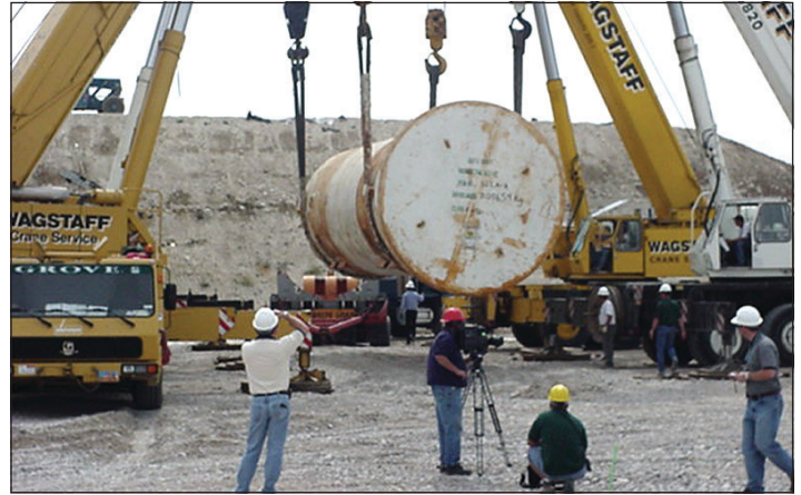
Large Component Disposition Disposal at EnergySolutions' Clive disposal facility in Utah's West Desert
